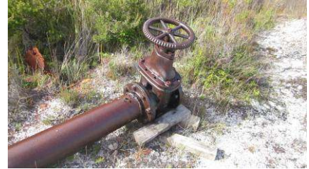
Well-oiled gate-valve, a potential exhibit on the future mining trail. Photo: Janet Fenton
